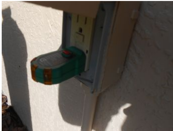
Exterior GFCI Reset in Bathroom #3
