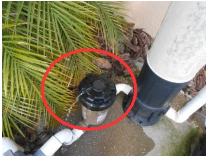
Chlorinator leaks at top when valve is moved
