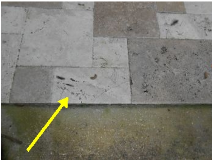
Cracked Tiles At Entry Way
