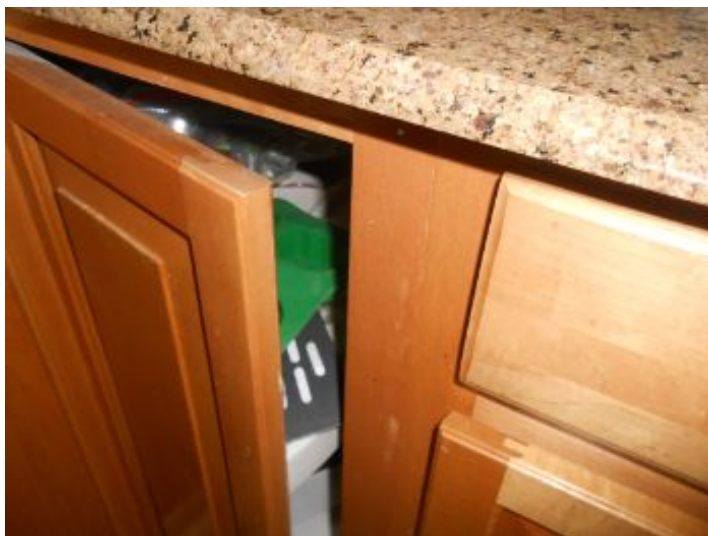
corner cabinet is difficult to operate
