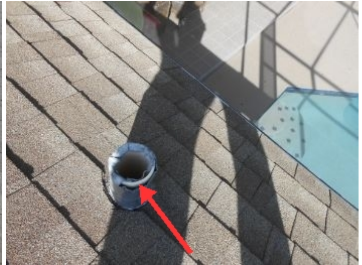
Damaged flashing boot
